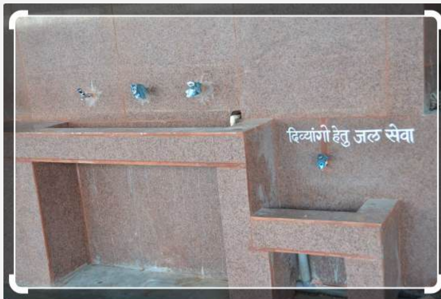
Picture of one of the drinking water facility installed with the help of NGOs
